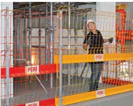
With the help of the post extension and a second mesh barrier, the edge protection can be increased to a height of 1.75 m.
